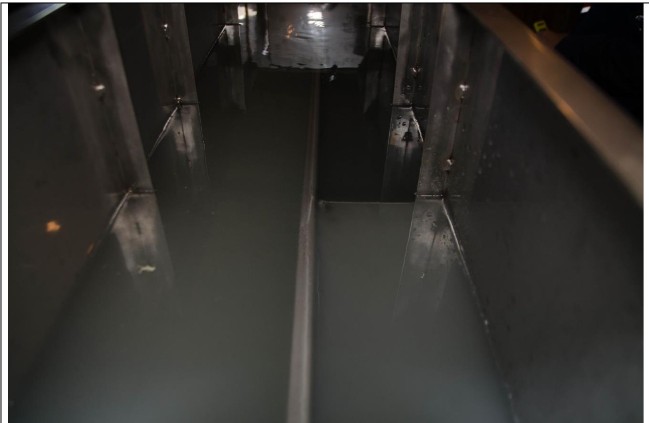
Figure 3: Feasibilitytest Industrial wastewater purification testfacility (sulphuric acid neutralization)
